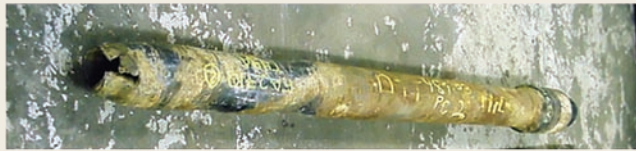
Downhole portion of failed joint
