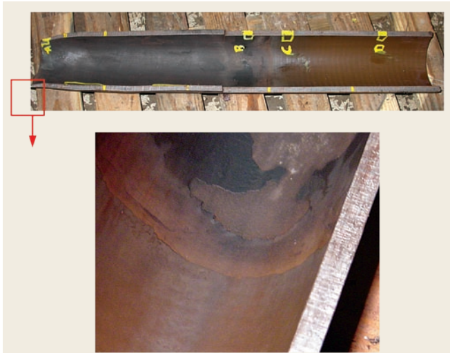
Fig. 5. Damage to internal plastic coating of joint C1 from exposure to high temperatures.
